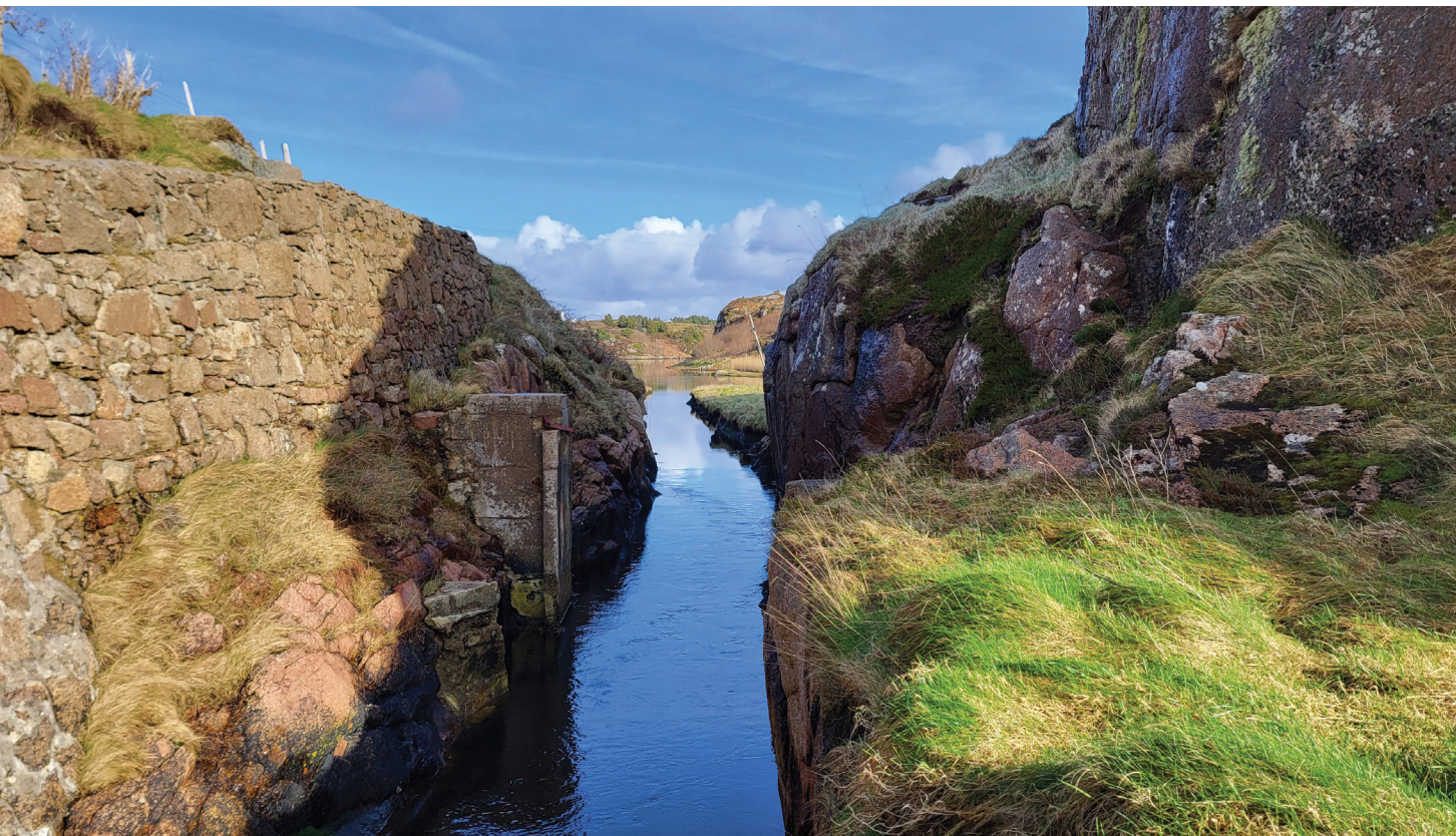
Figure 8.6 Sluice in the channel from Sally's Lough, County Donegal. Photo: Emer Magee
