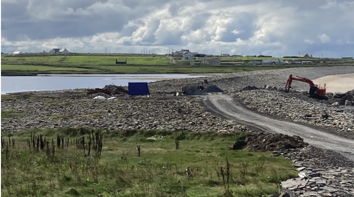
Figure 8.3 Lough Donnell showing management work being carried out on the barrier in 2023. Photo: Geoff Oliver
